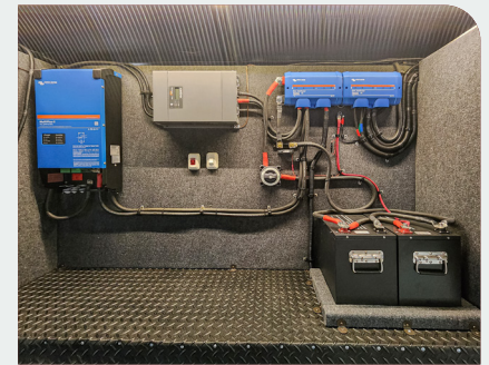
We give great attention to detail in our safety-minded approach to electrical wiring.
