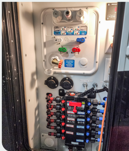
Utility center's residential manifold water system includes shut-offs for each fixture, black and gray tank flush-outs and dump valves.
